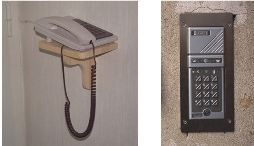
Figure 13 and 14. The access telephone placed in the hallway of a flat and the access telephone placed outside the entrance door of the building.
